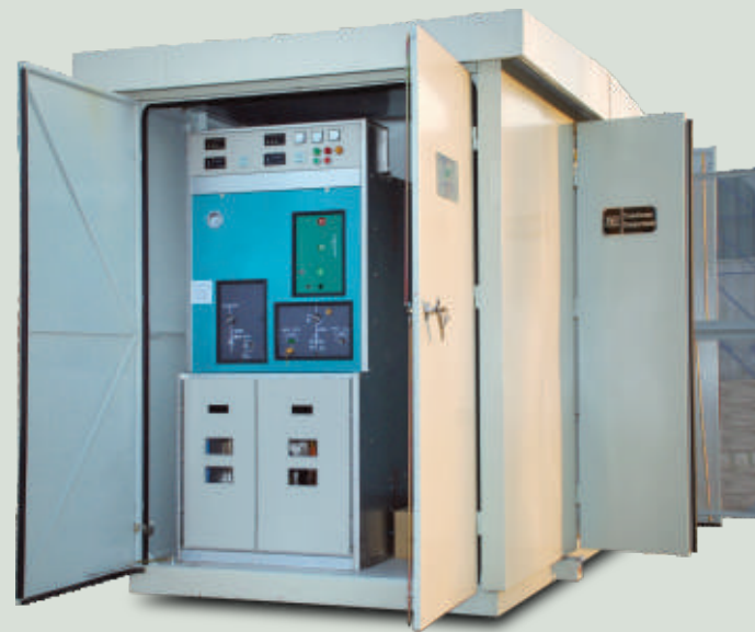
View of USS from HT Compartment side
