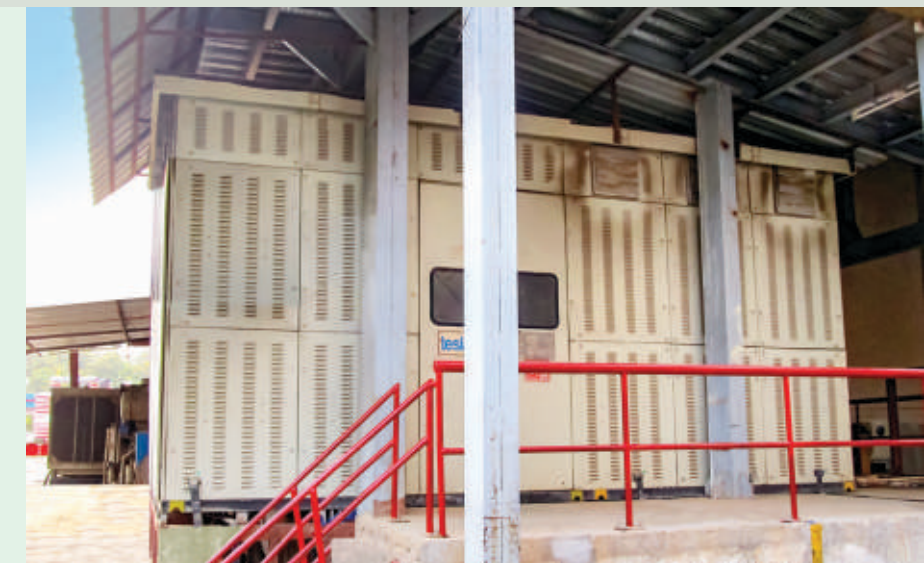
Tesla supplied 2500 KVA 33/0.433 KV USS with Cast Resin Transformer and GIS installed at Aura Mall Bhopal
